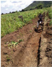
Excavation of land for the ongoing fencing of the One-hectare plot for ESN National Secretariat in Abuja
